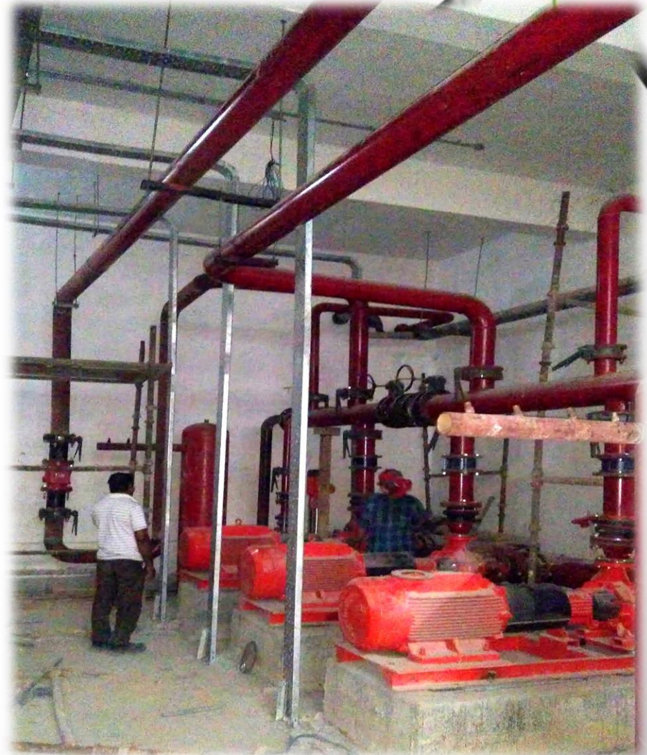
Pump House Metro Station 137 Noida
