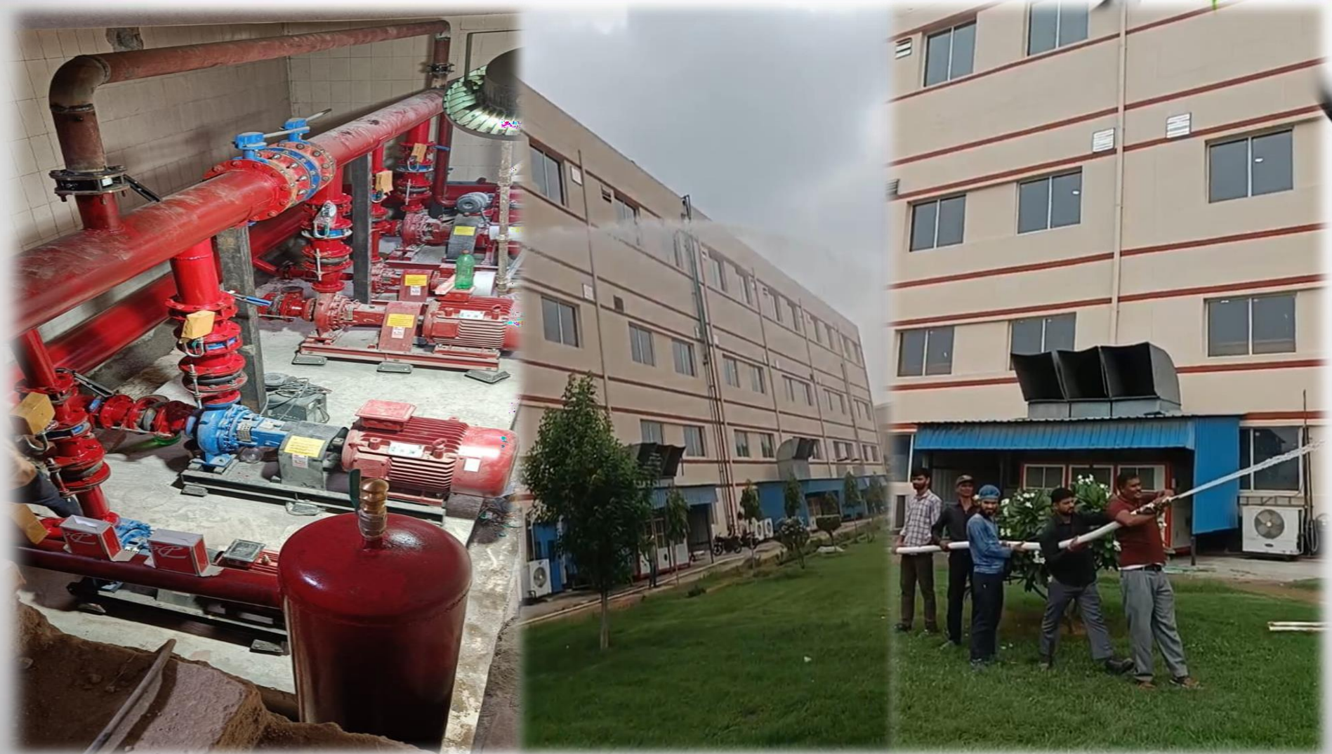
Fire Mock Drill & Fire Pump House Dharuhera Site Rewari Haryana
